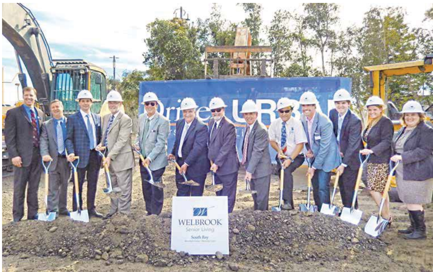
Welbrook Senior Living held a groundbreaking of its newest community, Welbrook South Bay, located at 3210 W. Sepulveda Blvd. in Torrance. Specializing in independent living, assisted living, memory care, skilled nursing and transitional care, it will feature 70 apartment homes scheduled to open in late 2014. Pictured (L to R) are Welbrook Principle Partner Matt Rasband, Principal Partner Ken Magargee, Principle Partner Doug Brawn, Torrance Councilman Pat Furey, Principal Partner Dr. Vince Valdez, Torrance Mayor Frank Scotto, Councilman Kurt Weideman, Councilman Tom Brewer, Councilman Bill Sutherland, Capital Senior Housing Founder & Managing Partner Scott Stewart, VP Kyle Henderson, Integral Senior Living COO Collette Valentine and Divisional VP Mandy Hampton. Photo by Charlene Nishimura.
